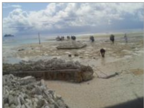
Boat ramp totally destroyed in Nanumaga Island
