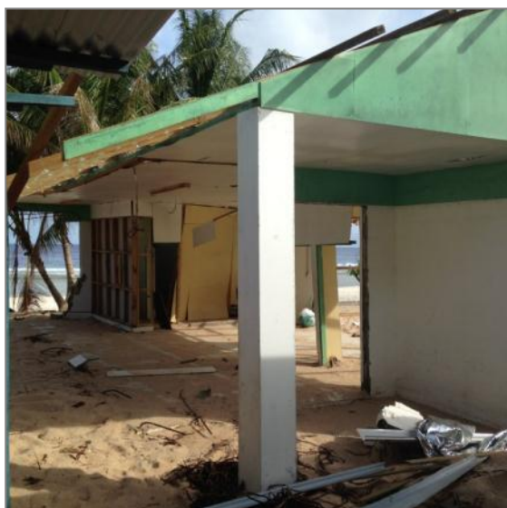
Damaged clinic in Nanumaga: Courtesy of Red Cross
